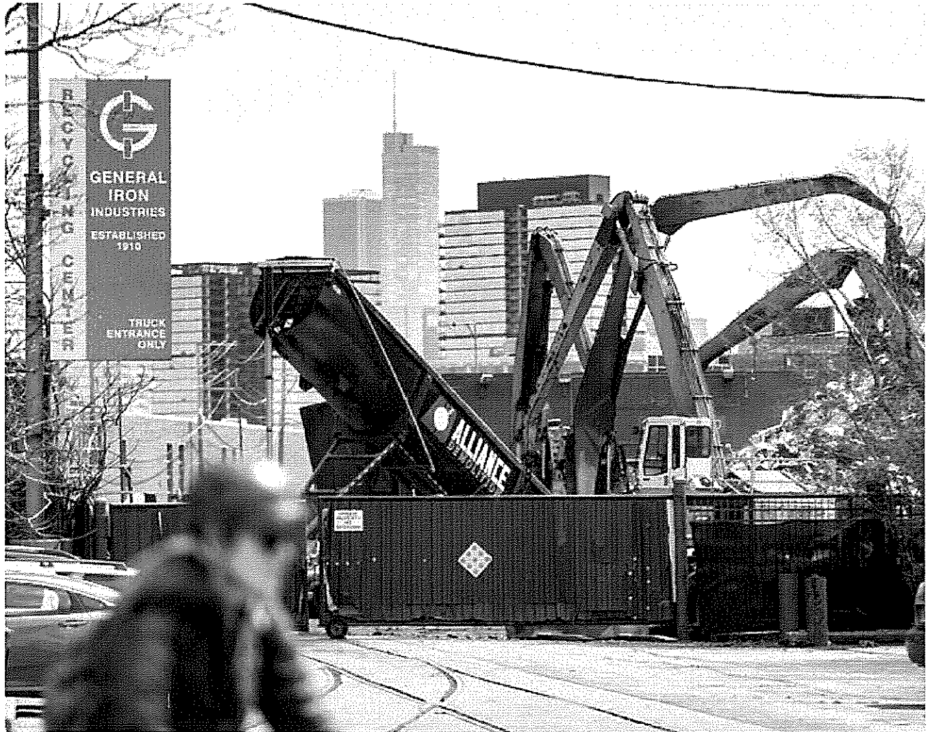
General Iron Industries scrap yard at work along Cortland Street near the Lincoln Yards development is shown on April 9, 2019.(Brian Cassella / Chicago Tribune)
